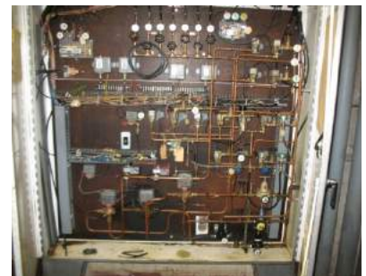
Pneumatic Controls Station - Image 3
