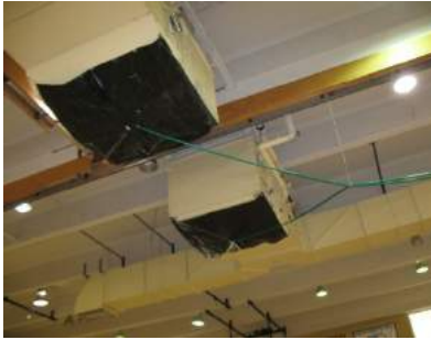
Gymnasium Fresh Air Hood Leaking - Image 10
