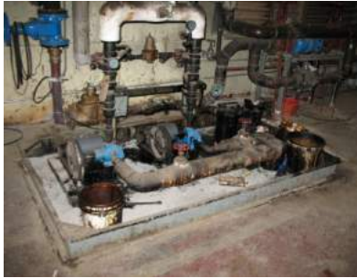
Fuel Oil Transfer Pumps - Image 5
