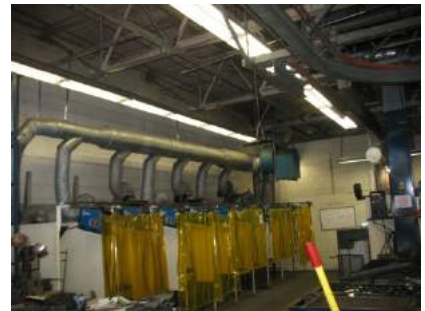
Welding Booth Exhaust - Image 13
