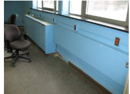
Typical Unit Ventilator & Finned Tube Radiation – Image 7
