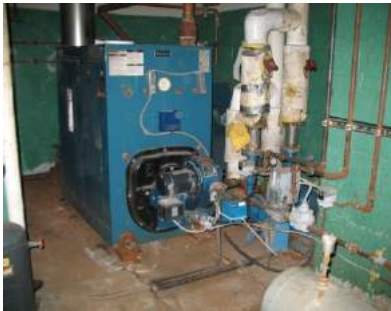
Pool Heating Boiler - Image 11
