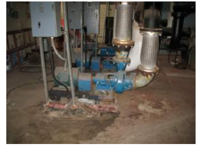
Chilled Water Pumps - Image 1
