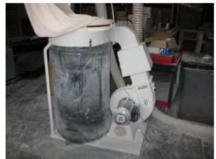
Carpentry Shop Local Dust Collector - Image 14
