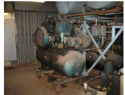
Duplex Controls Compressor - Image 2
