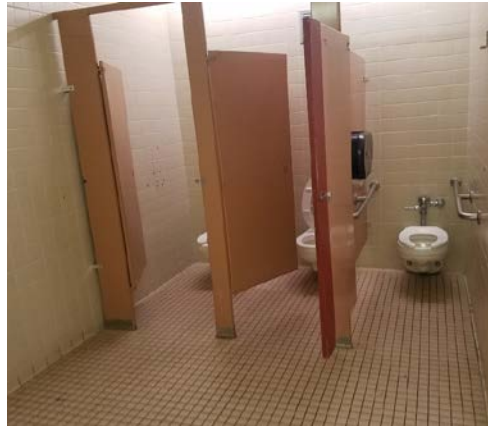
Toilet stalls too small and grab bars noncompliant.
