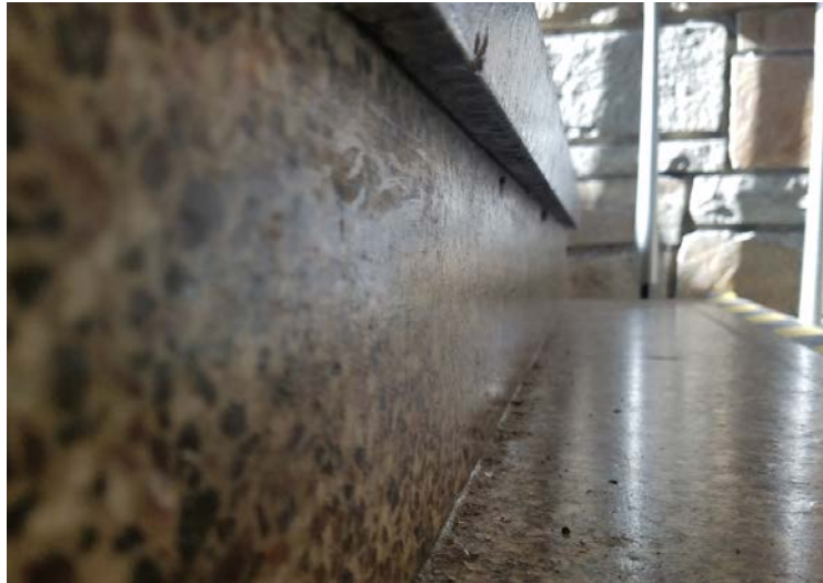
Abrupt nosing on stair.
