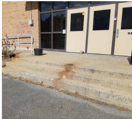
Stair is missing a handrail.
