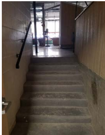
Stair is missing a handrail.
