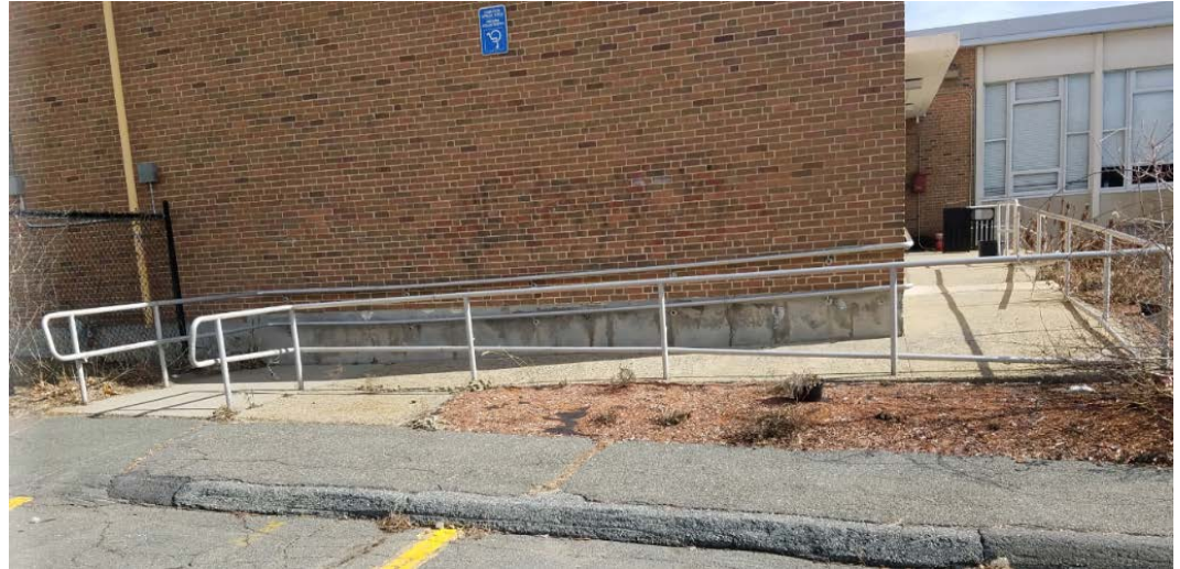
Handrail are not compliant and the ramp has a cross slope larger than 2%.
