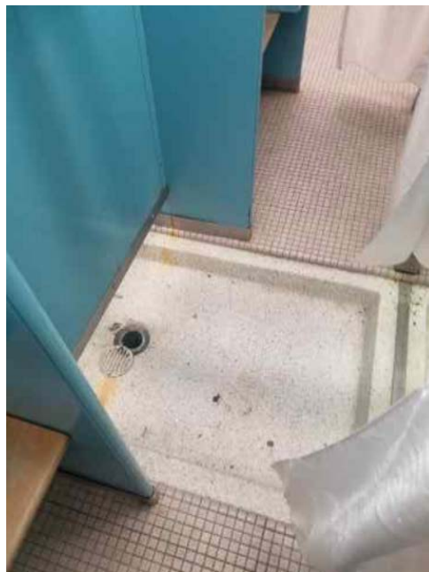
Shower is too small and has a barrier.
