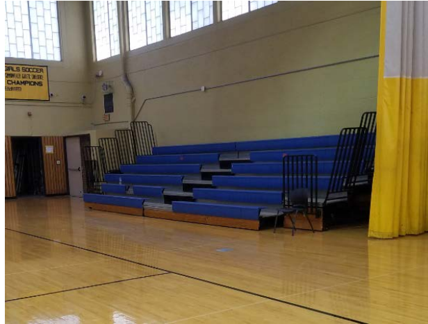
Bleachers are missing handrails in the aisle.
