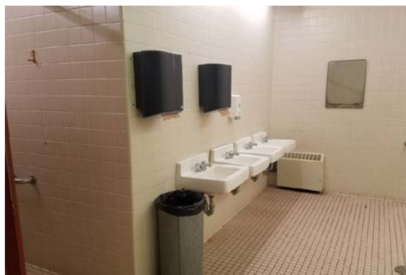
Sinks not compliant.
