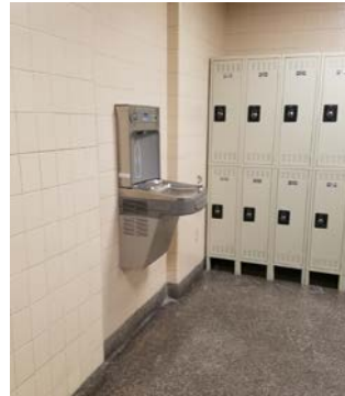
Protruding into the corridor more than 4 inches.
