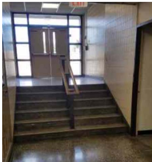
Stair is missing handrails on the sides.
