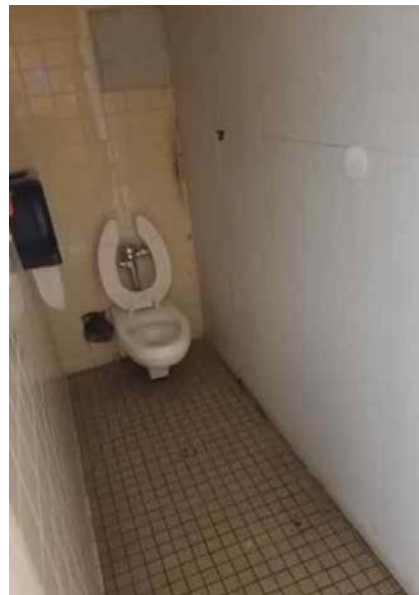
Stall too small and no grab bars.
