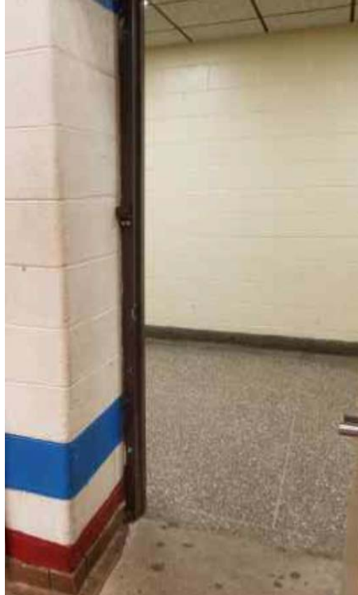
Door does not meet clearances.
