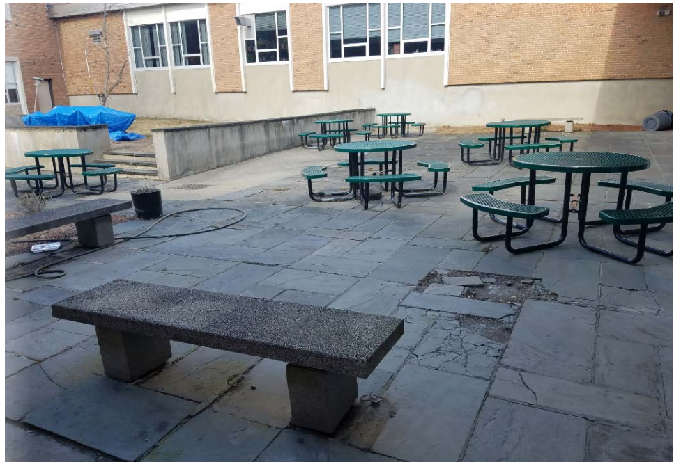
Stairs to the raised portion of the courtyard and concrete in disrepair.
