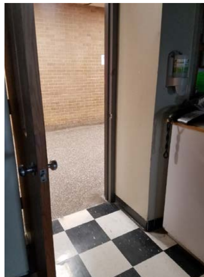
Door does not meet clearances and has doorknob.
