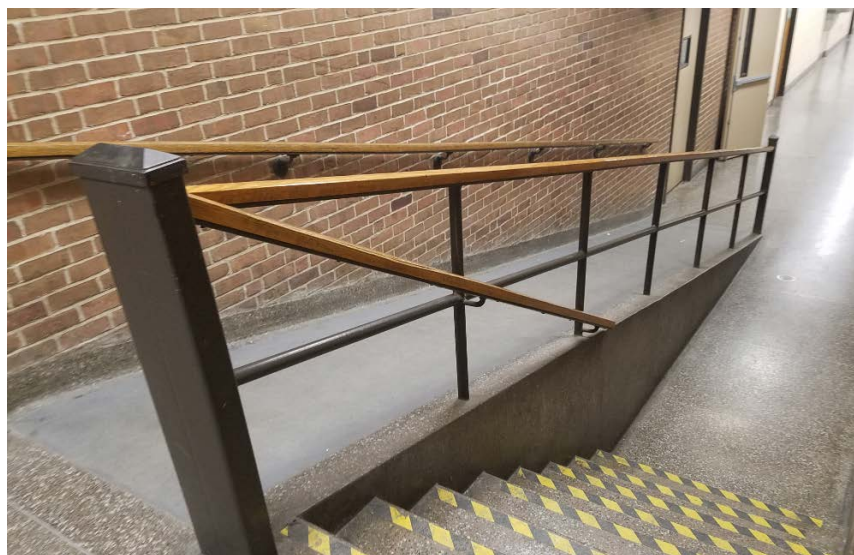
Steep ramp over 8.3% slope. The handrails are noncircular and do not extend.
