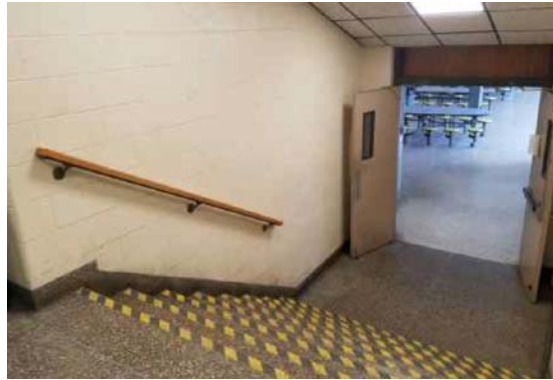
Handrail is noncircular and does not extend at the top or the bottom.
