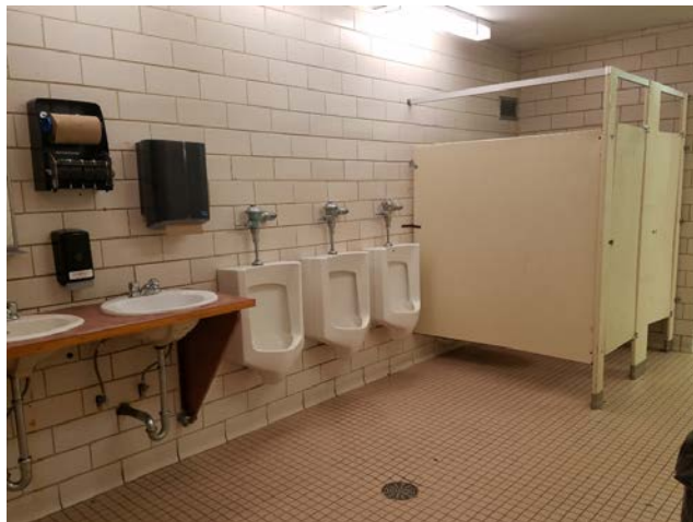
Toilet stalls too small, urinals too high, and sinks not compliant.
