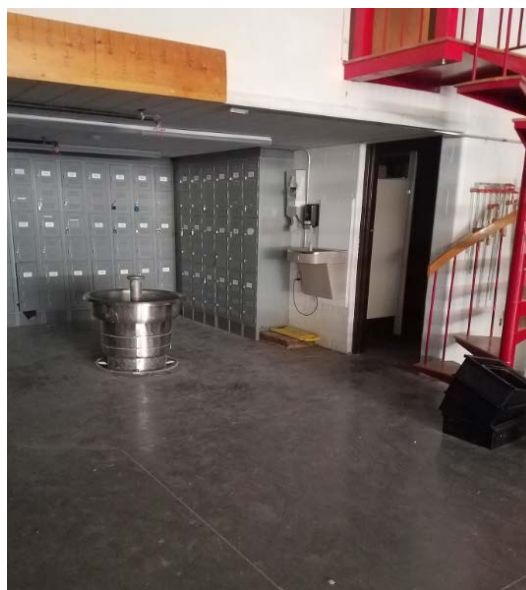
No accessible route to the upper level and non-accessible sink.
