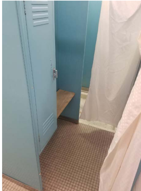
Changing area is noncompliant.
