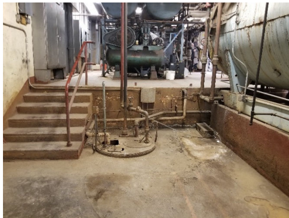
Existing deficient Sump Pump and Basin
