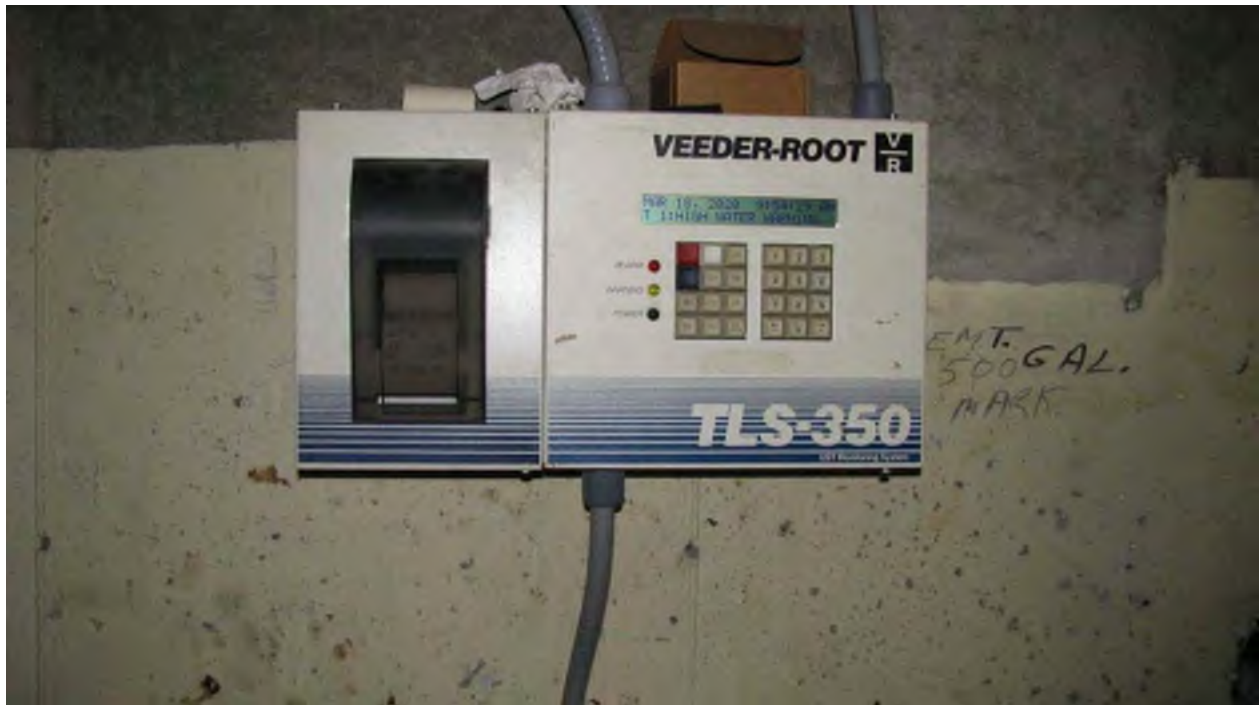
Photo 23. View of the leak detection monitor for the 20,000 gallon #4 fuel oil UST.
