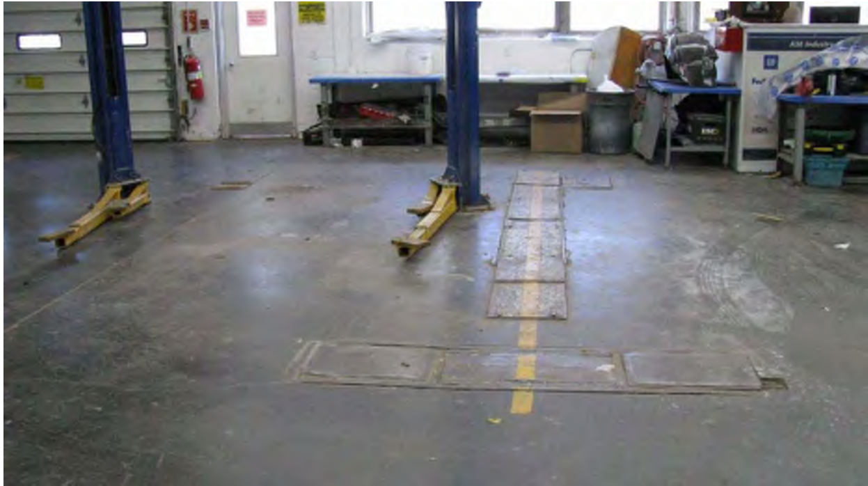
Photo 17. View in the Auto Mechanics Shop of typical electric aboveground lifts currently in use and former underground hydraulic lifts no longer in use.
