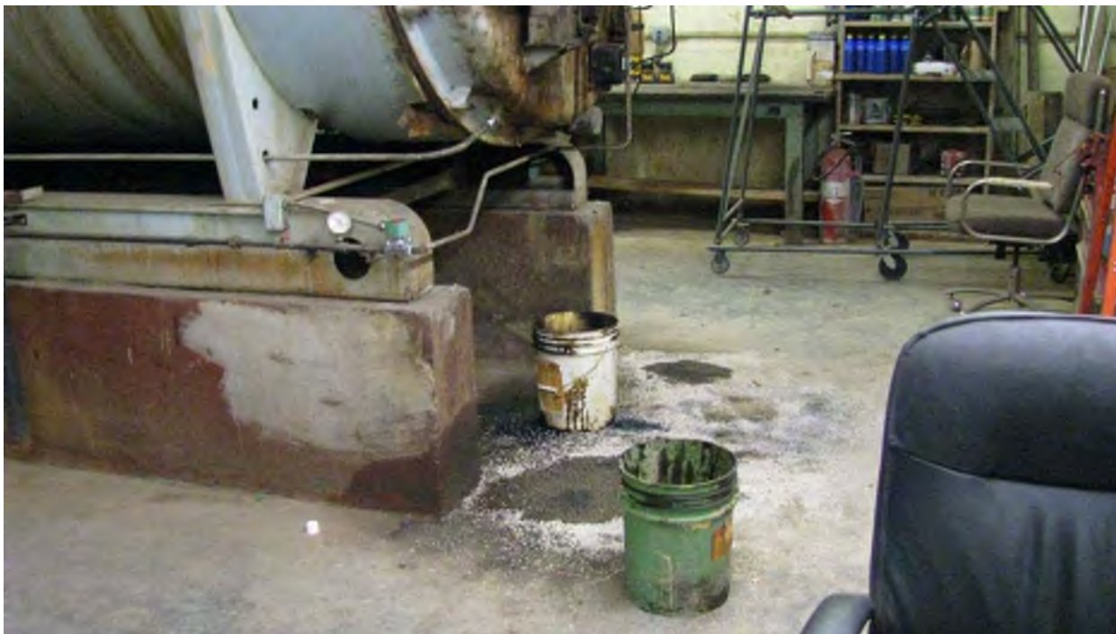
Photo 22. View of a hot water boiler in the Boiler Room.
