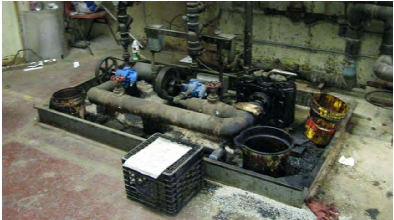
Photo 24. View of containment for the fuel oil transfer pumps in the Boiler Room.
