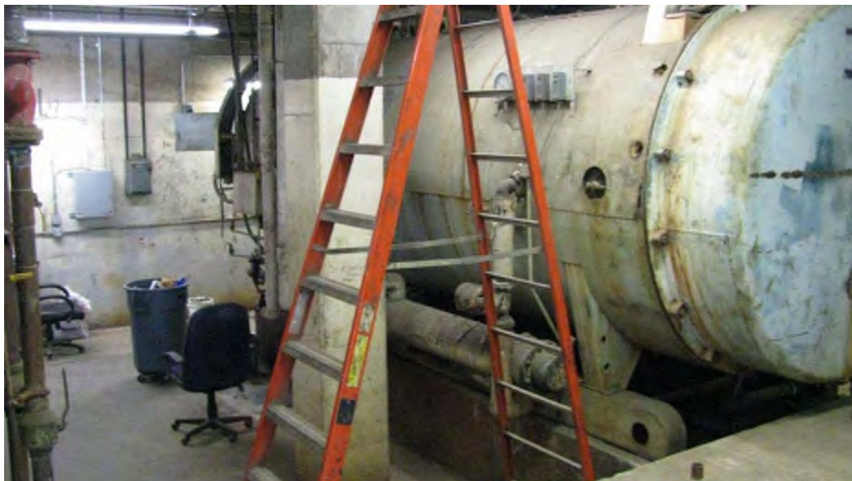
Photo 21. View of a hot water boiler in the Boiler Room.
